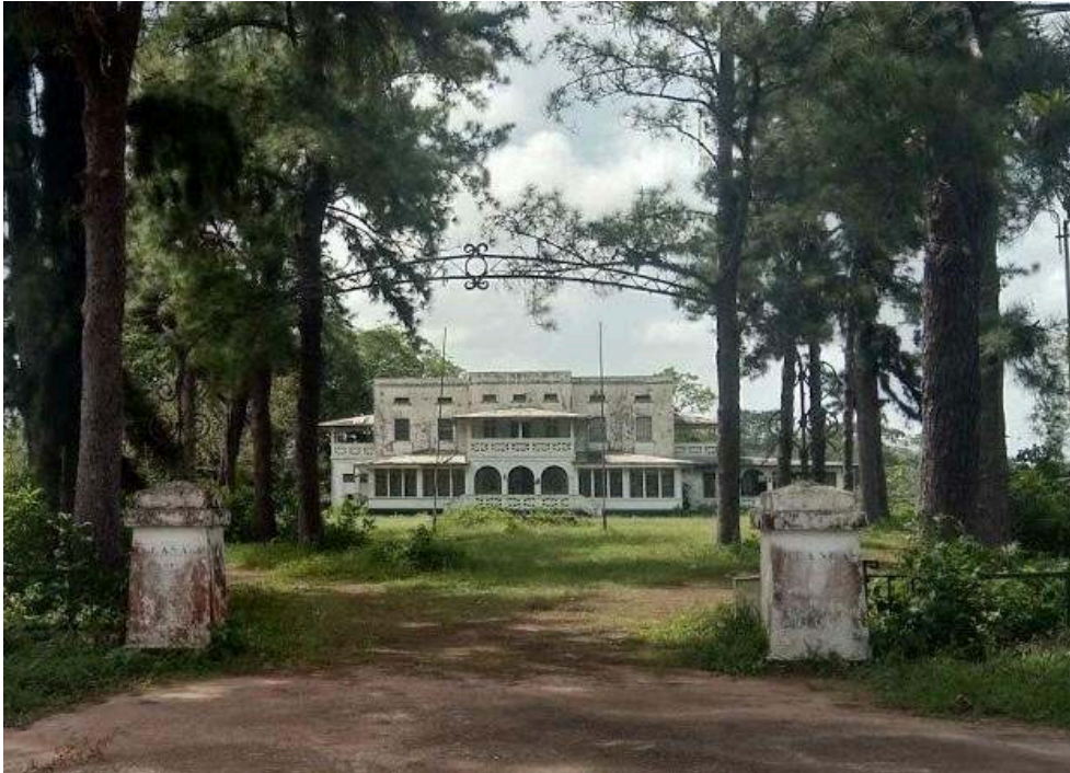
Figure 2.2 The Casa Blanca, Moengo's guesthouse, pictured in 2020 in a state of disrepair
